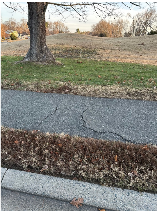
Roots and cracks near #1 golf course hole
