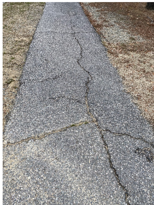
Cracks and grass/weeds
