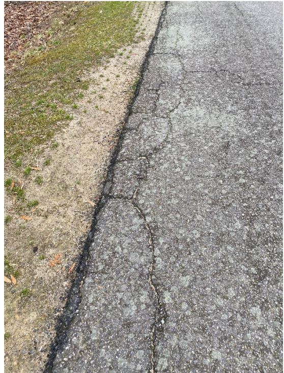
Edge drop-off &amp; cracks near Birkdale Golf Club
